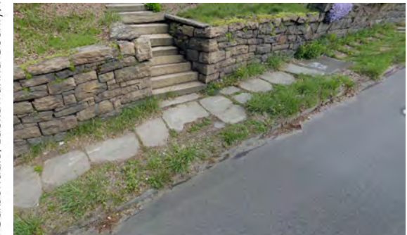
Example of “Poor” Sidewalk Condition
