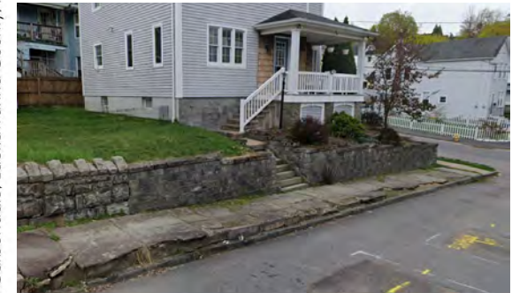
Example of “Poor” Street Curb Condition
