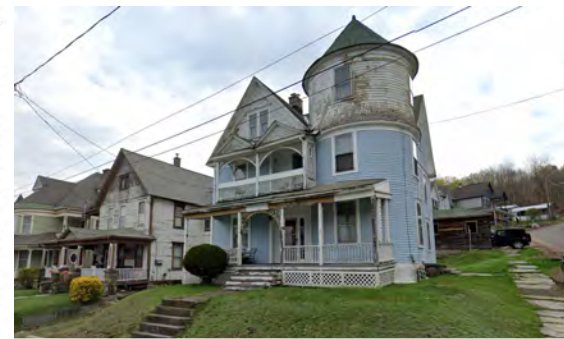
Example of “Poor” Façade Condition
